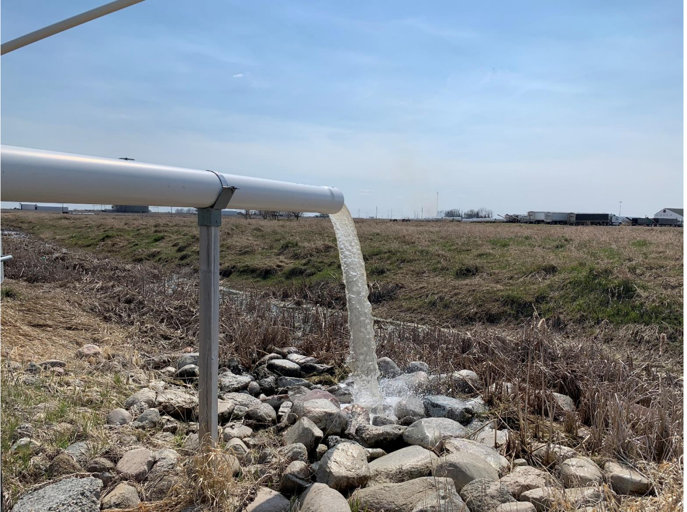
Figure 1. The NDSU Langdon Research Extension Center Groundwater Management Research Project Lift Station.
