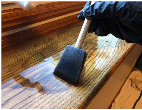
Fig. 3 Oxalic acid solution was applied to the stain with a foam brush. The solution was applied twice and resulted in lighter, but still visible, stains.
