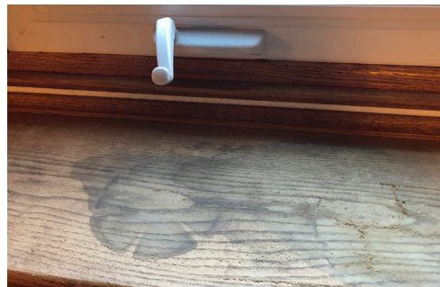
Fig. 1 This area in front of the window shows evidence of black water stains from potted plants. The stain on the left shows the wedge outlines of a plastic protective tray.
