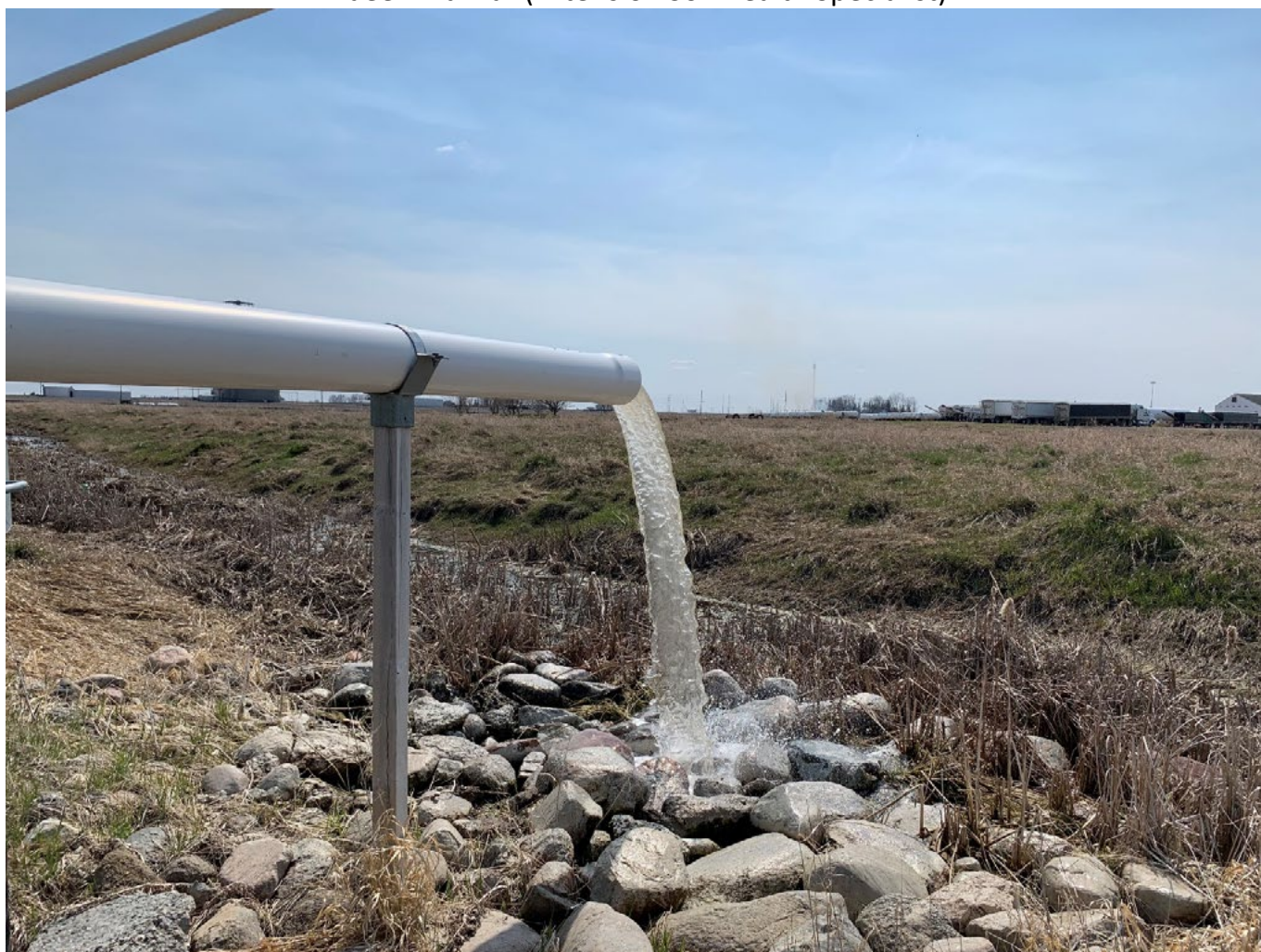
Figure 1. The NDSU Langdon Research Extension Center Groundwater Management Research Project Lift Station.
