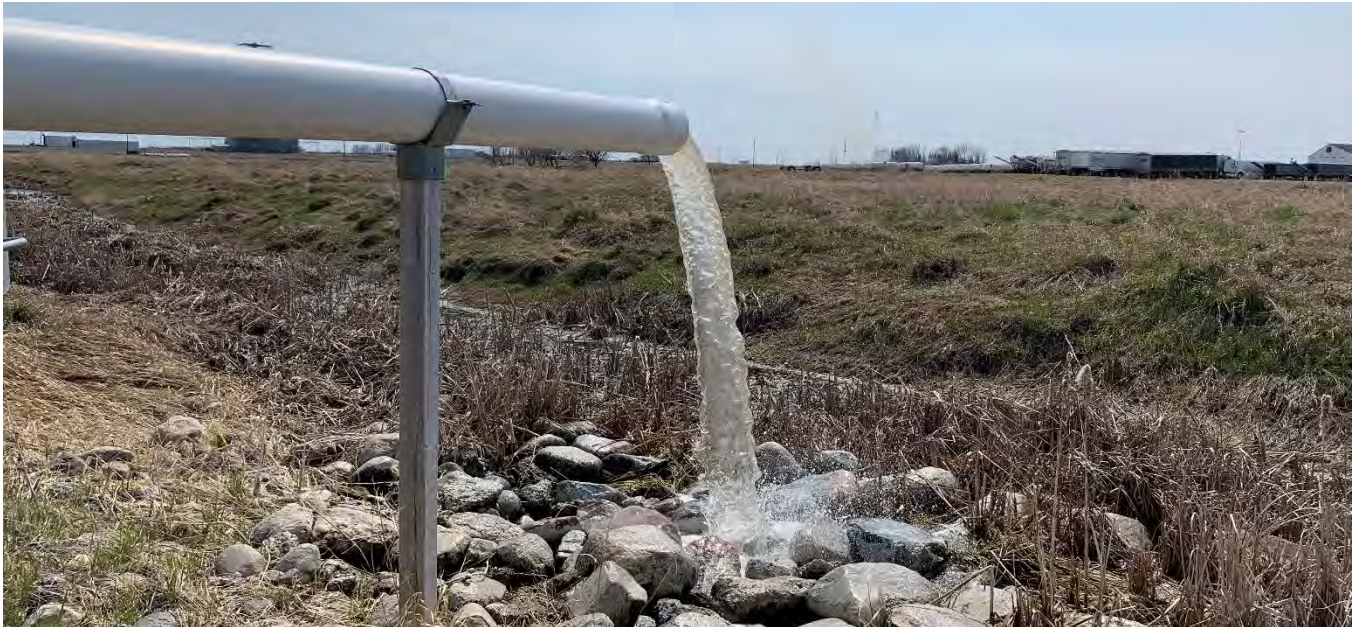
Figure 1. The NDSU Langdon Research Extension Center Groundwater Management Research Project Lift Station.
