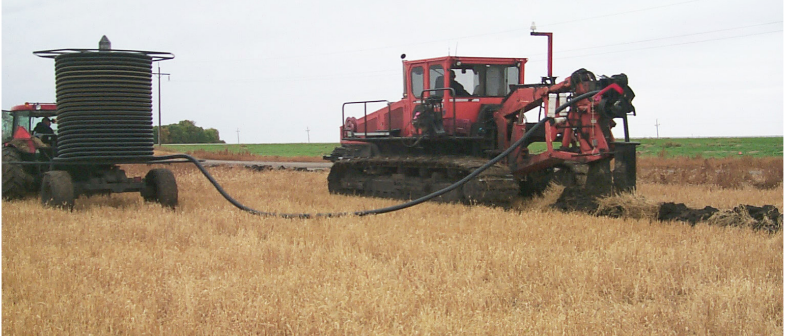
Figure 11. Installation of tile drainage in progress in Ramsey County along state Highway 17 near Edmore, N.D. (Photo courtesy of Ronald Beneda, NDSU Cavalier County Extension agent).
