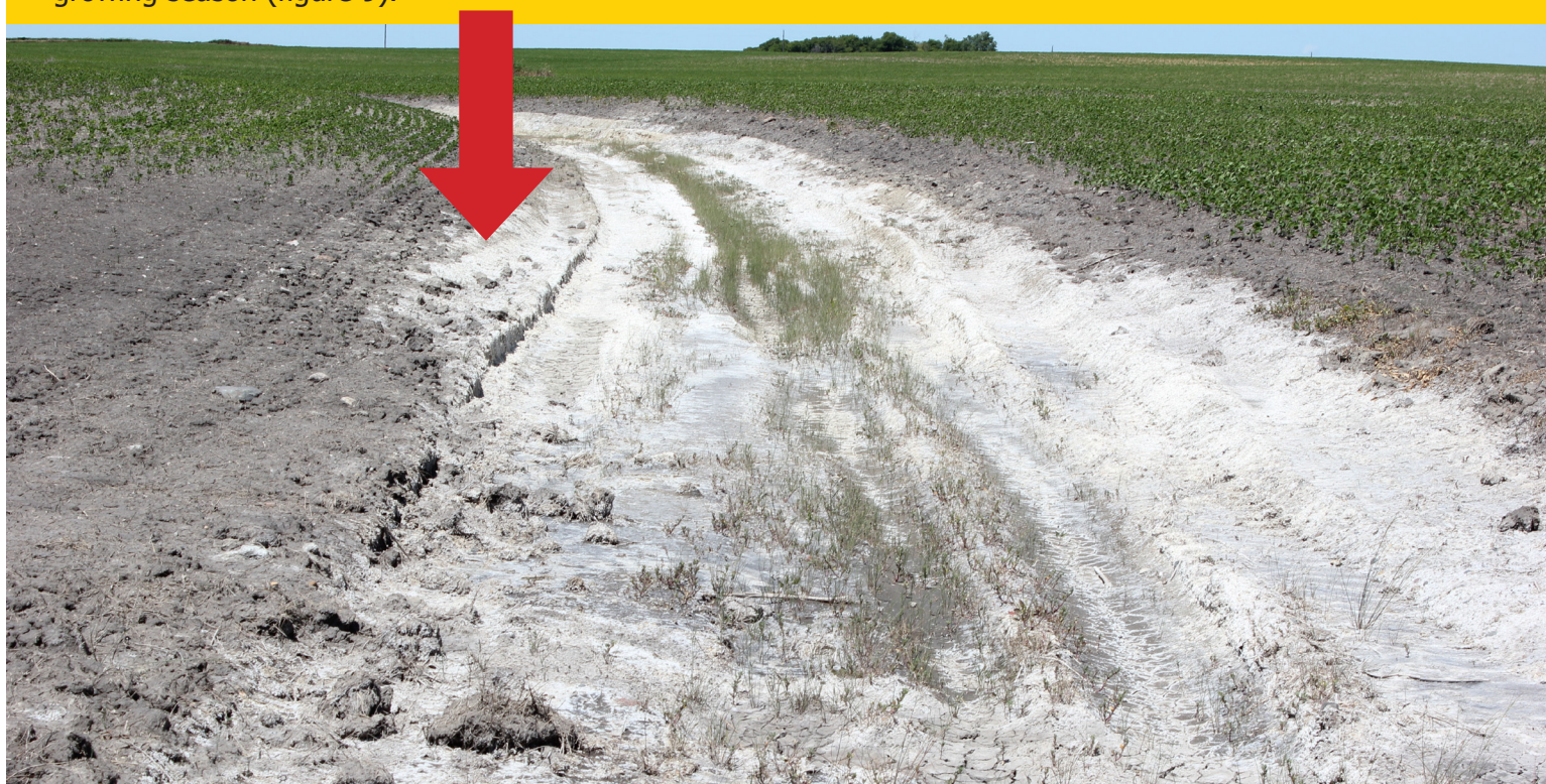
Figure 9. A field ditch, acting as a shallow pond during the growing season along state Highway 17 near Edmore, N.D.
